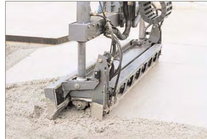
Concrete parking delivers speed and lower installed cost: Concrete pavement technology is continually improving. Laser screeds speed up placement time, improve accuracy and reduce labor costs.
